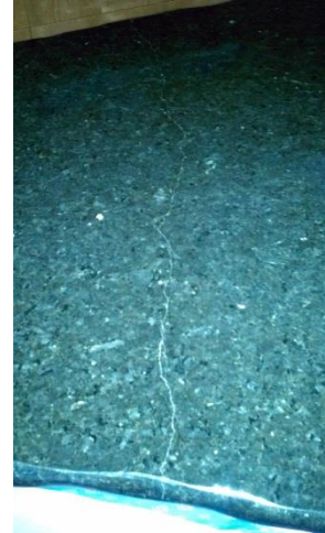
Granite crack created by thermal stress.
